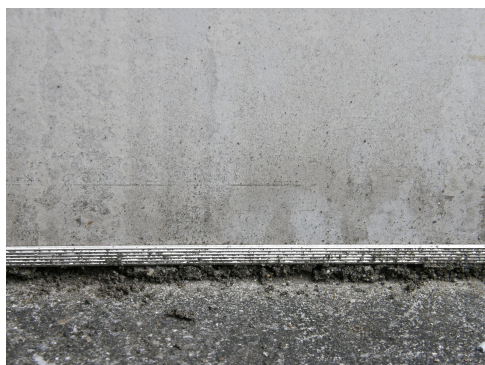
Photo 3. Gap between the Wall and Floor on the Roof Sand accumulated in the Gap.
